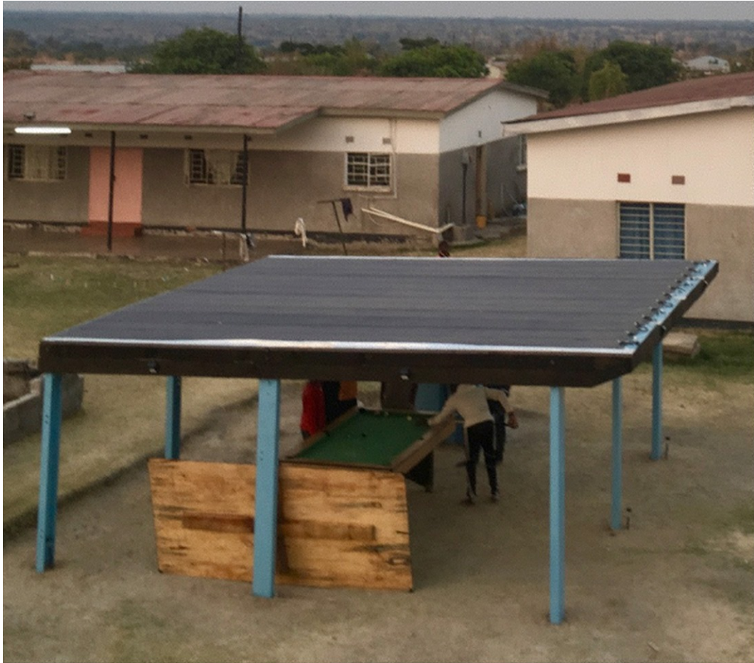
FIGURE 5.2 Photograph of build in Mutende, Lulamba, Zambia with twelve 136 W amorphous Si PV panels with an inverter/charger for two 102 Ah lead acid batteries feeding a mains outlet. A small DC system powers internal lighting (six LED bulbs) a radio and two USB charging points through a small battery bank.
