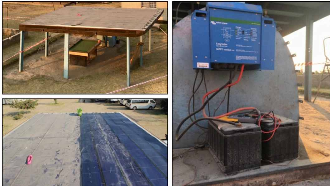
FIGURE 5.9 Photographs of the build in Mutende, Lulamba, Zambia 12 months after installation, demonstrating the problem dust can cause on PV systems in challenging climates. Dust accumulation on PV modules (left) and batteries and inverters, even in enclosed spaces (right), is a major problem.
