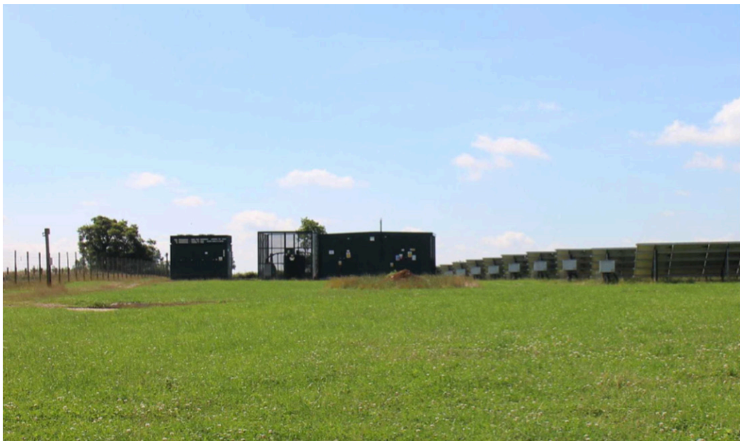
FIGURE 19.9 Solar farms include transformers, CCTV cameras and fences as well as panels. Dorset, UK. Photo: B. Dower (all rights reserved).
